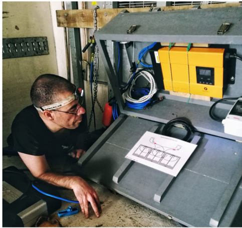
FIGURE 4 A pure sine wave inverter converted 24 V DC (or 12 V DC) from a truck (or van) to 220 V AC, which powered the filtration units on all the tanks [Color figure can be viewed at wileyonlinelibrary.com ]
